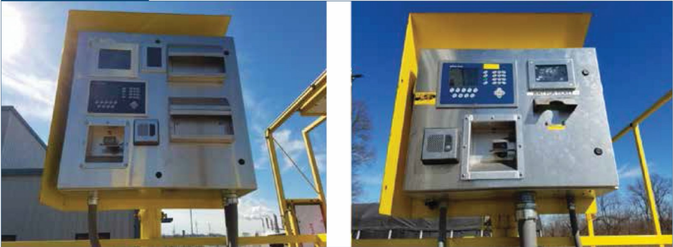
Scale kiosks. Nucor Steel Gallatin has an inbound scale, an outbound scale and one bidirectional scale. Any of the scales can be put into or taken out of service by the flip of a switch.
